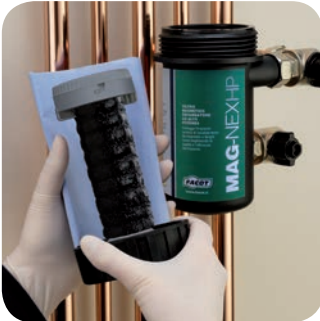
Figure 5 - Magnet impregnated of magnetic sludge
